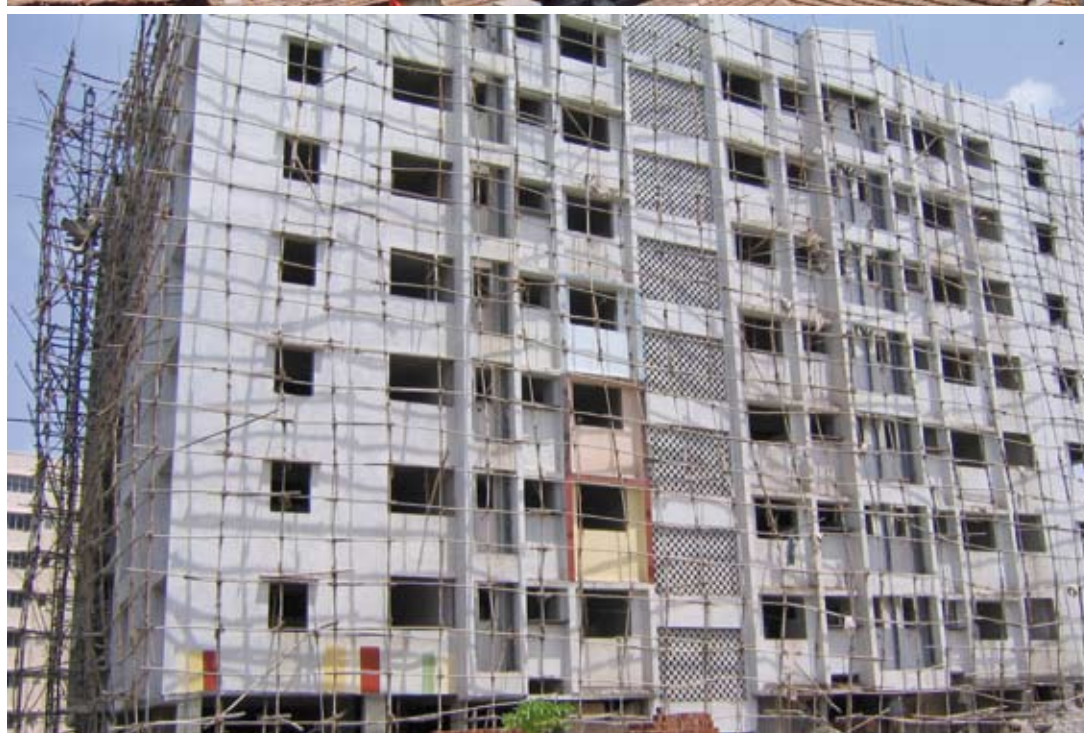
Nouvelle construction à Bharat Janta, dans le bidonville de Dharavi. New housing in Bharat Janta, in the Dharavi slum.
